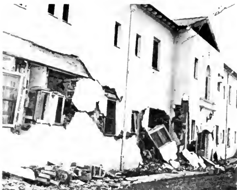
Photo 47. Partially collapsed building having hollow clay tile filler walls, Veterans Administration Hospital. Los Angeles County Fire Department photo.
